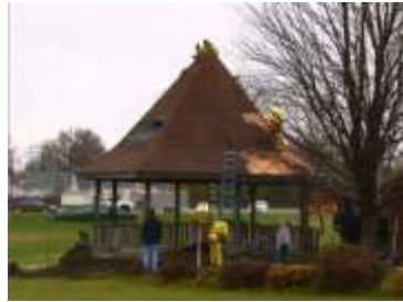
Volunteers spent the day rebuilding ramps and railings, along with repairing the gazebo's roof. (Source: WOIO)
