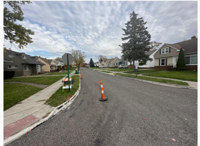
Pictured above, construction underway of Longview Avenue. This road was resurfaced this fall.
